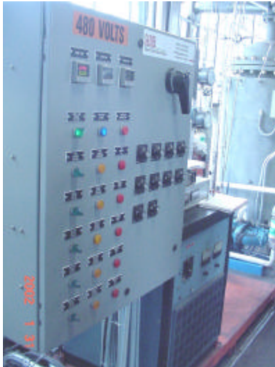
Figure 11. Control Panel and Power Supply
