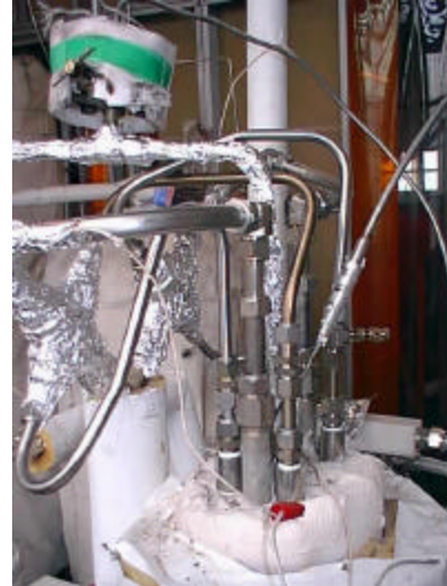
Figure 12. Feed and Overflow Lines
